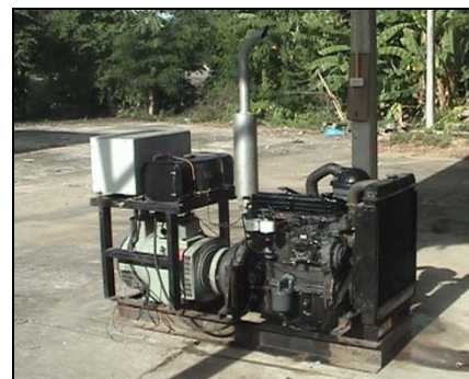
Fig.1 25 kilowatts diesel generator set
